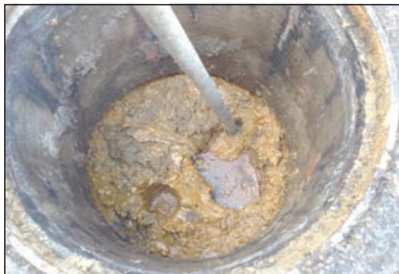
Fat, oil and grease accumulation in a sanitary manhole. Improperly disposed cooking grease and so-called flushable wipes create costly system challenges.
